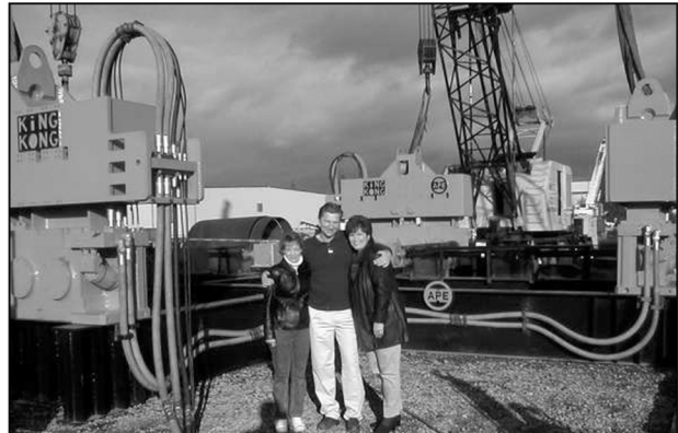
Wendy Setlege, wife of Randy Setlege, President of Agra Group and John and Teresa White stand in front of the "Quad Kong" which is four APE Model 400 vibratory driver/extractors mounted together to install 40 foot diameter concrete pipe piles in China.
