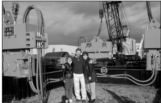
Wendy Setlege, wife of Randy Setlege, President of Agra Group and John and Teresa White stand in front of the "Quad Kong" which is four APE Model 400 vibratory driver/extractors mounted together to install 40 foot diameter concrete pipe piles in China.
