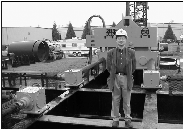
Jack Xu, Managing Director for APE China, stands on Caisson beam of Quad Kong System, Dec. 2001.
