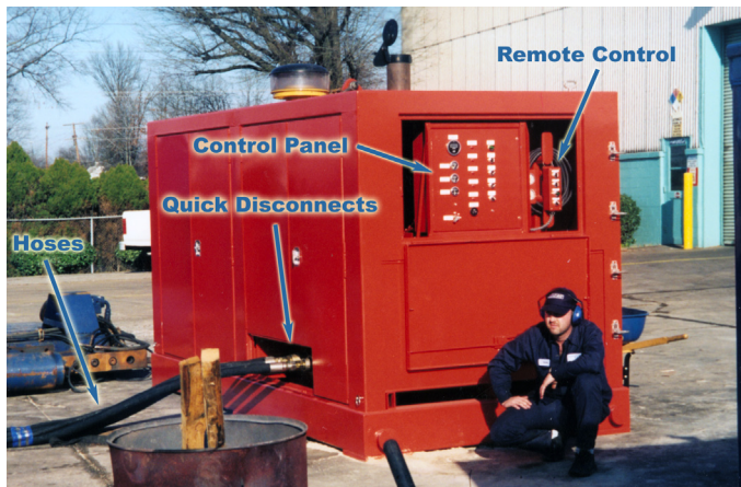
Figure 3-66 External View of a Power Pack
