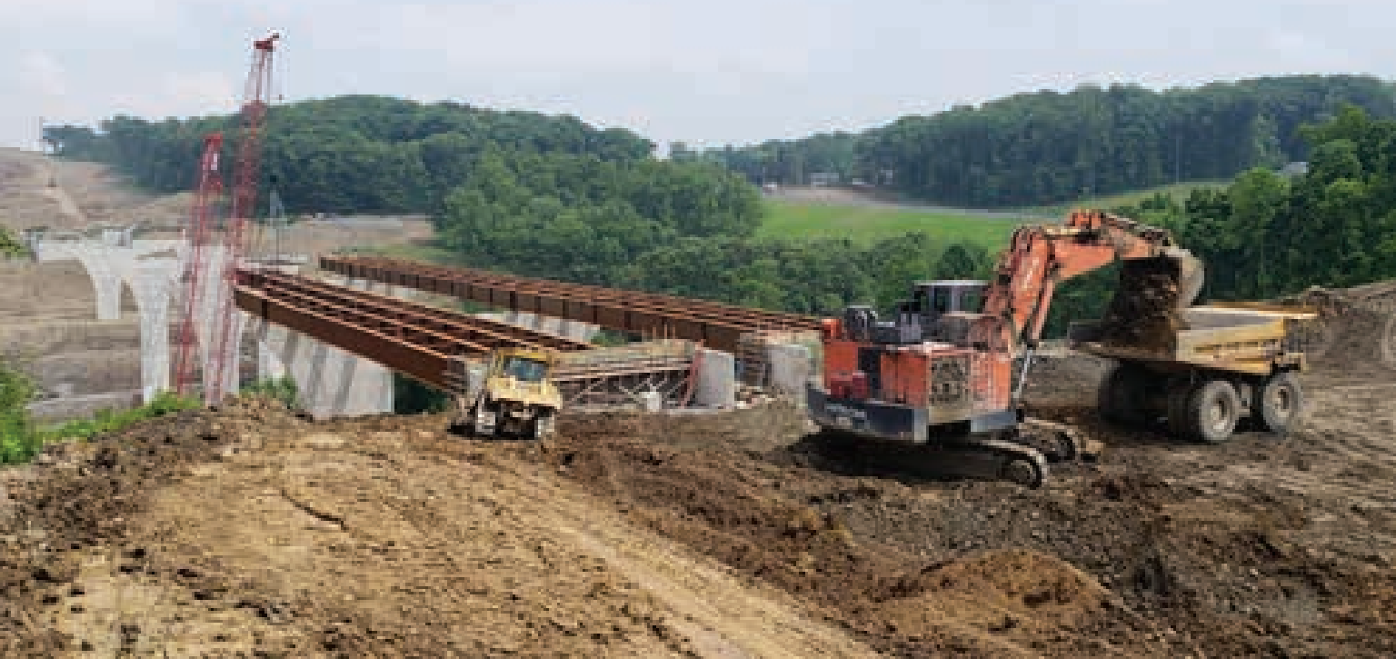
Close up of mass excavation completion on the west side of the SR980 bridge structure. Shows the Hitachi 1900 Excavator with 777 Truck, D8 shaping slope configuration, and erection of the Dual Span Bridge structures utilizing two 2250 Manitowoc Cranes.
